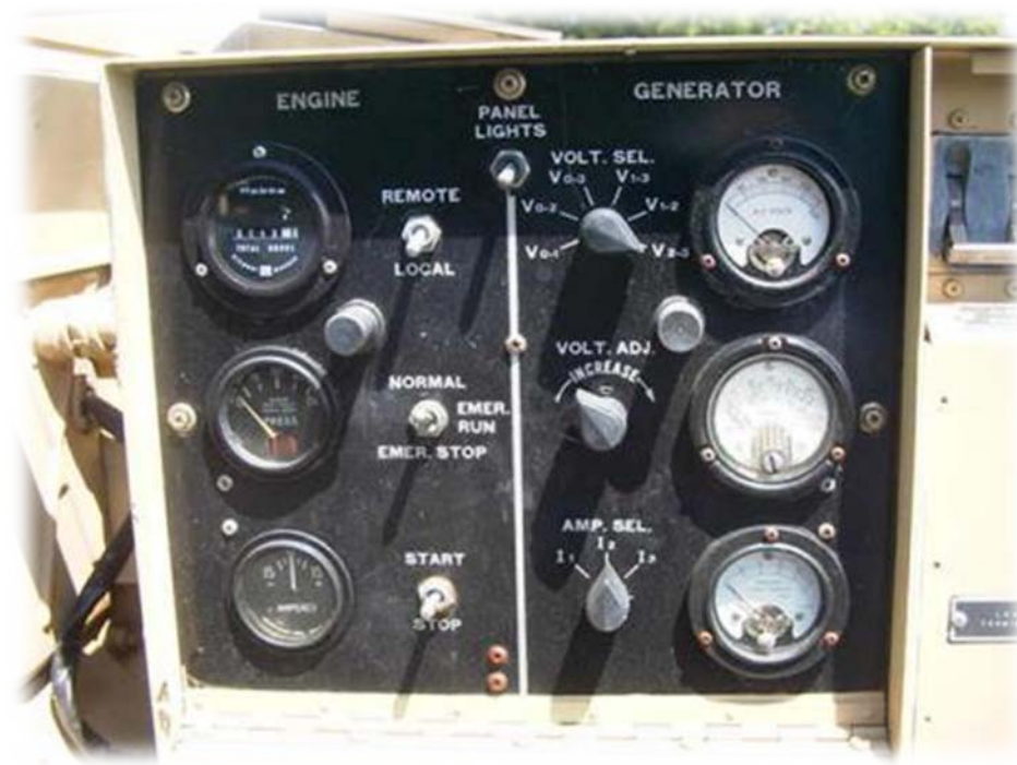
Figure 7 MEP-017A Control Panel Instrumentation - photo by author
